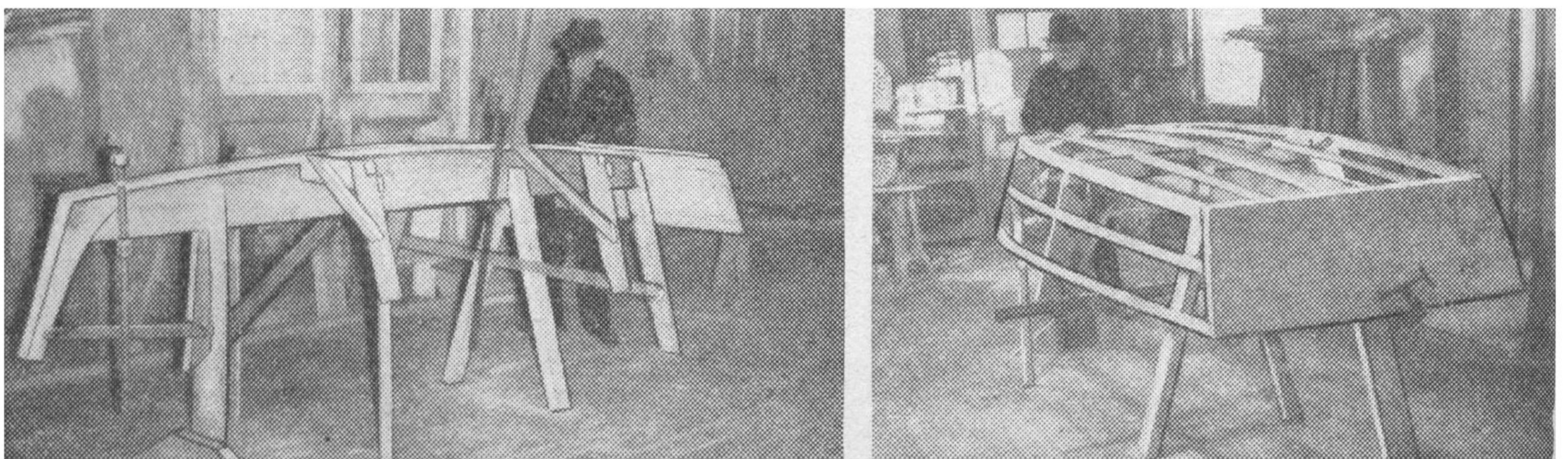
Left, form with temporary molds in place. Right, framework completed with transom in place.
