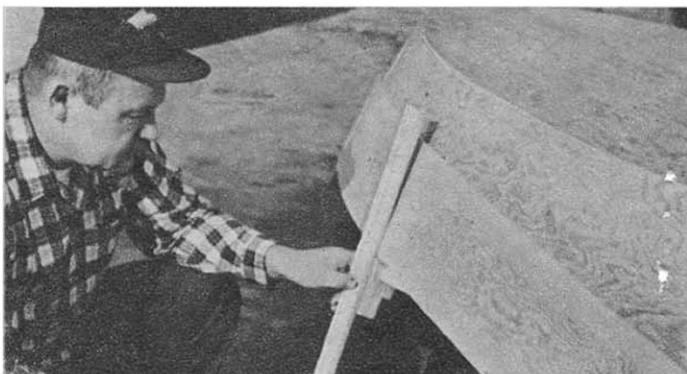
SECOND STRAKE should fit flush into frame notch. Check, then true up with hand plane.
