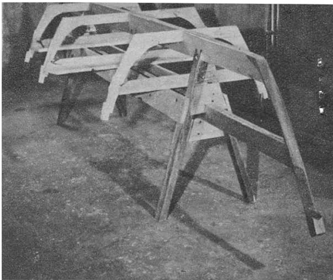
STEM, FRAMES, transom set up on building jig. Make sure 2 by 6-in. plank is well dried.
